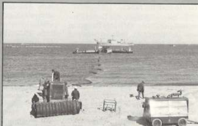
INSTALLATION of amphibious assault bulk fuel system. Omnipresent ORI evaluator is in white hat.
