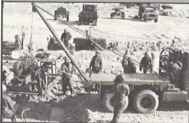
FUEL ELEMENT places power tong to begin pipe assembly for the bottom lay fuel system.
