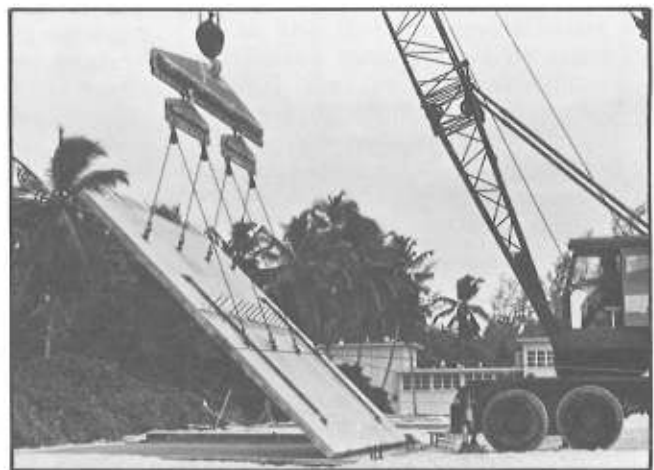
PRECAST PANEL is tilted into position as bulkhead for new bachelor's enlisted quarters on the Indian Ocean atoll.
