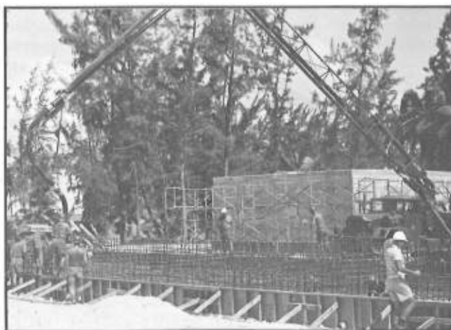
CONCRETE is pumped into foundation forms for 568,000 liters (150,000 gals.) water storage tank on Diego Garcia site.
